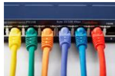
Figure: Network Cables
