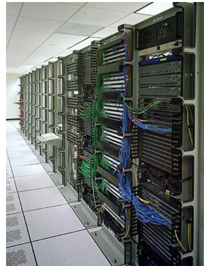
Figure: A Data Center
